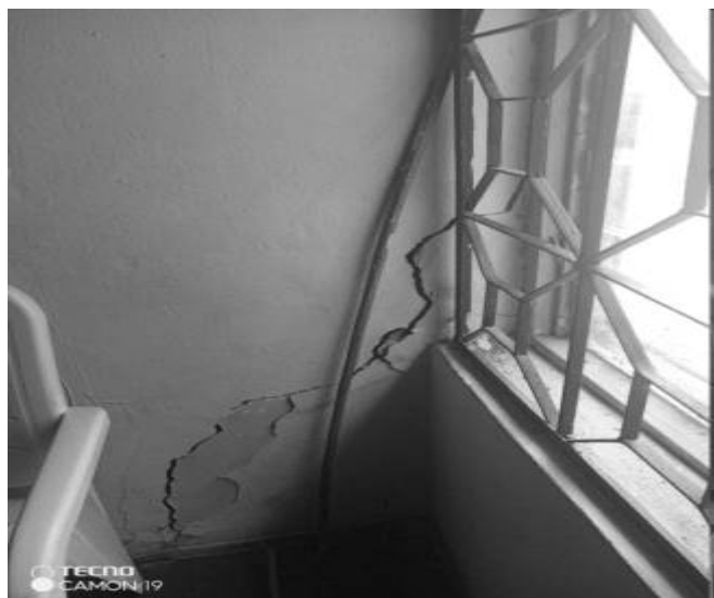
Plate9: The main office building needs an urgent intervention for rehabilitation
