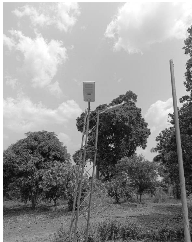
Solar street light in front of admin
